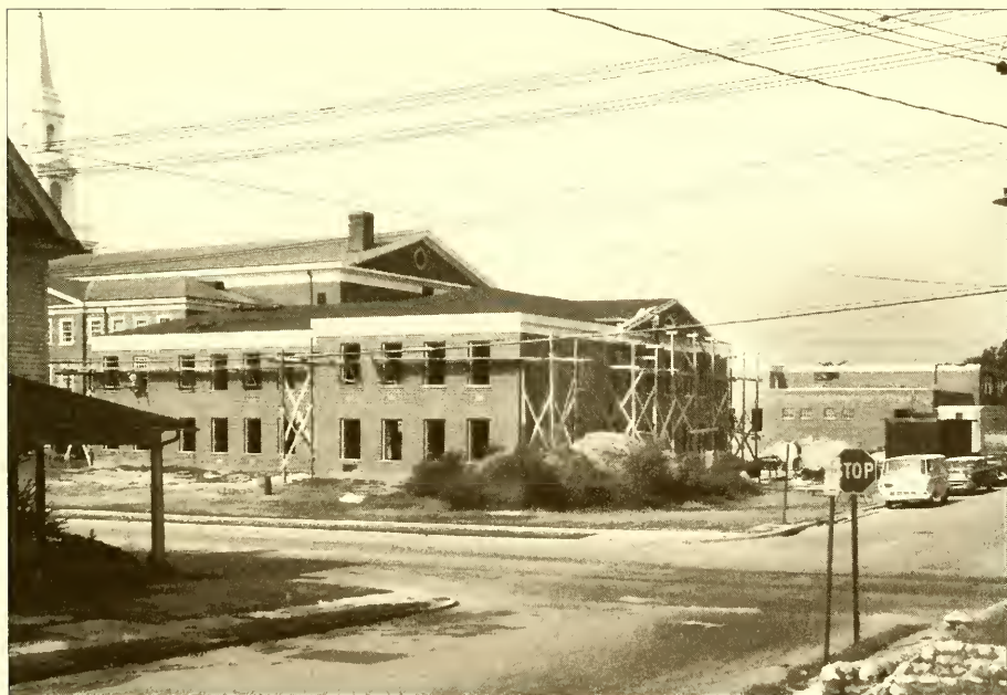
The educational space known as the children's wing was under construction in 1963.
